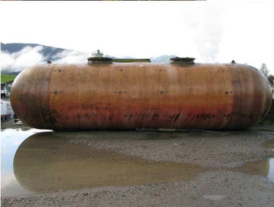
Buoyancy restraint strap guides are visible along the top half of the tank.
