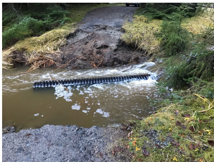
Figure 15 - Washed out driveway on Parker Drive
