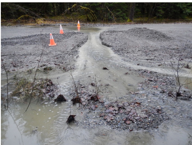
Figure 4 - Wilson Road Damage Near Dock Ponds Trail (December 2020)
